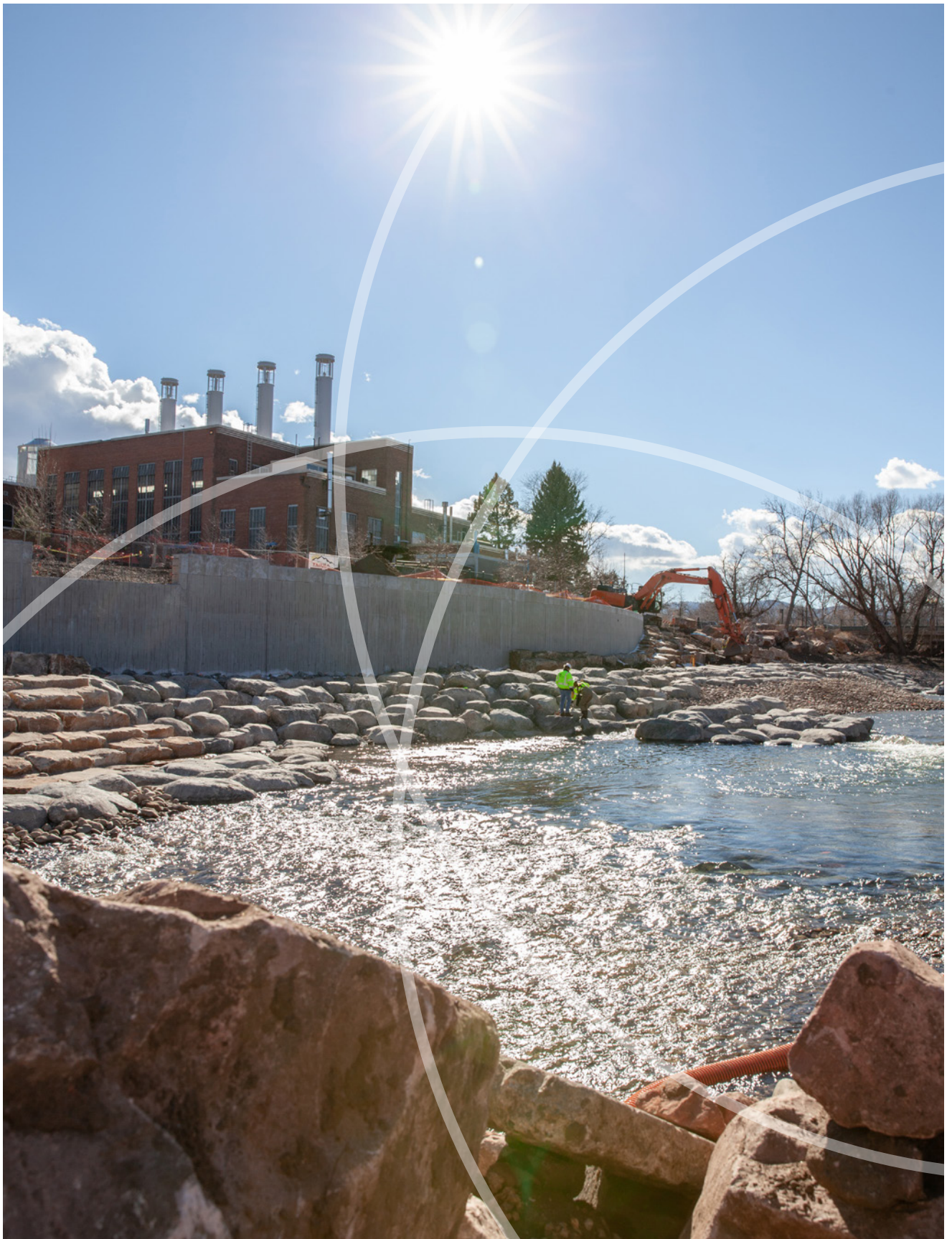
Construction of the Poudre River Whitewater Park, a project that will bring the river back to a more natural state and improve the river floodplain.
